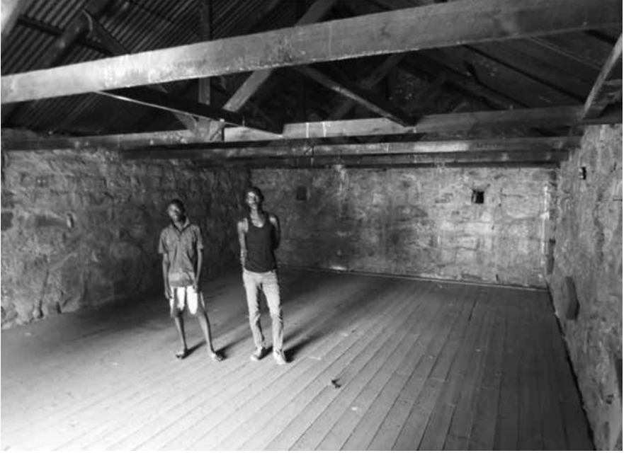
Interior of the closed loft, formerly a grain store, above the mill; note the splayed rafter-slits and condition of the floor
