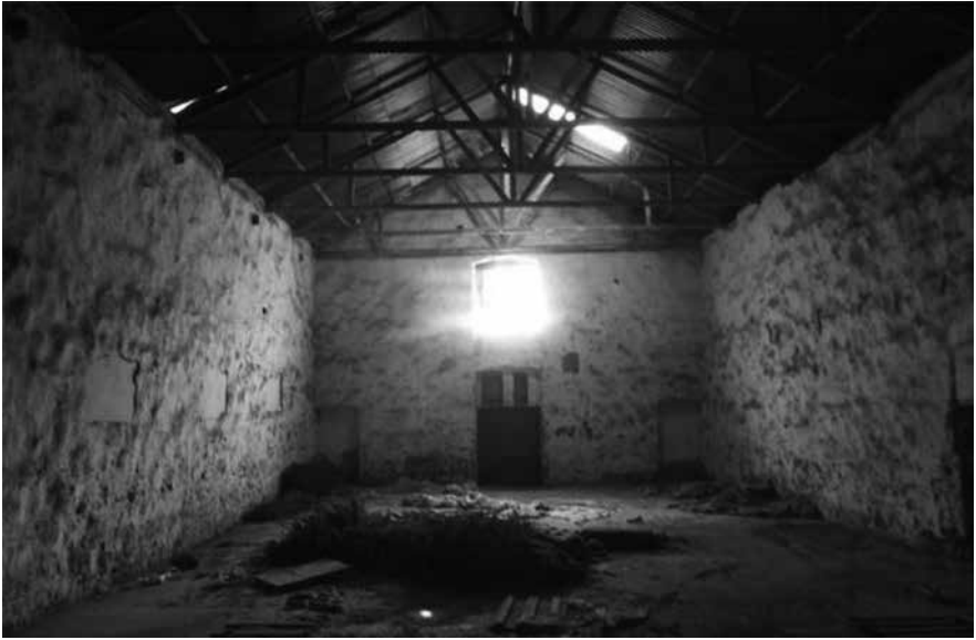
West looking interior of the Coaching Stables; note the bricked-in stable windows on the left and the small doors for feeding/watering the mules; the roof is not original
