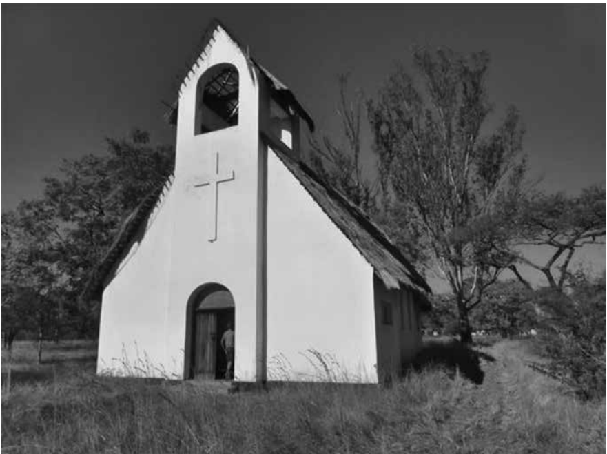
View from the west end showing the deteriorated state of the thatching over the bell-tower
