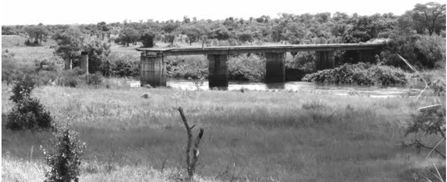
The remains of the bridge blown up by the Rhodesians. The object of the raid, codenamed “Operation Cheese”, was to make Zambia once again reliant on its southern transport links (Paul Hubbard)
