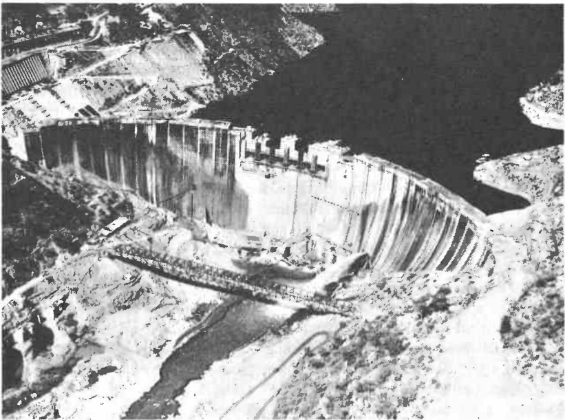
Kariba hydro-electric scheme: A general view of the dam wall, May 1959 (National Archives of Zimbabwe)
