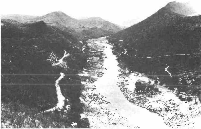
Aerial view showing dam site with coffer dam foundations in the left foreground looking downstream, August 1956
