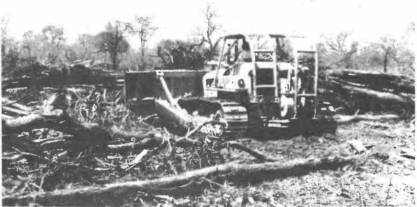
Bush clearing, Kariba basin: Euclid tractor pushing trees into rows, October 1958 (National Archives of Zimbabwe)
