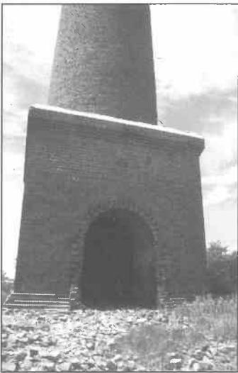
The base showing the arched opening into the former brick tunnel to the smelter.
