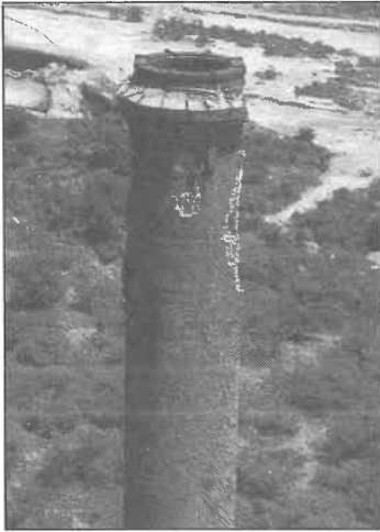
Exfoliation, with cracks progressing down the chimney.
